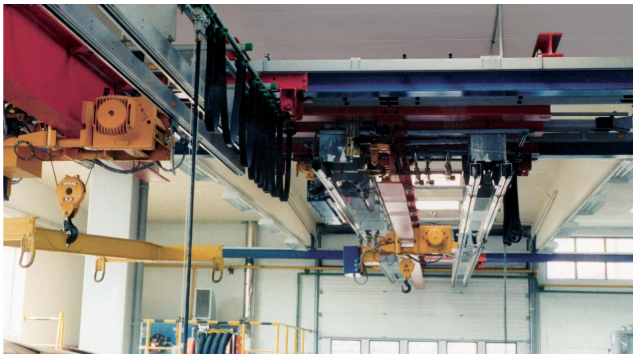
Aluminium enclosed conductor system on crane bridge.
