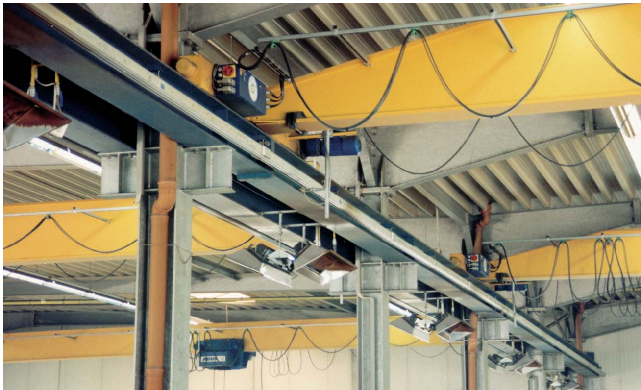
Aluminium enclosed conductor system for crane electrifications.
